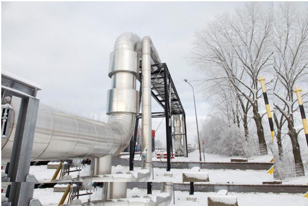
Figure A2: Current steam pipe from Twence to Nobian in Hengelo
